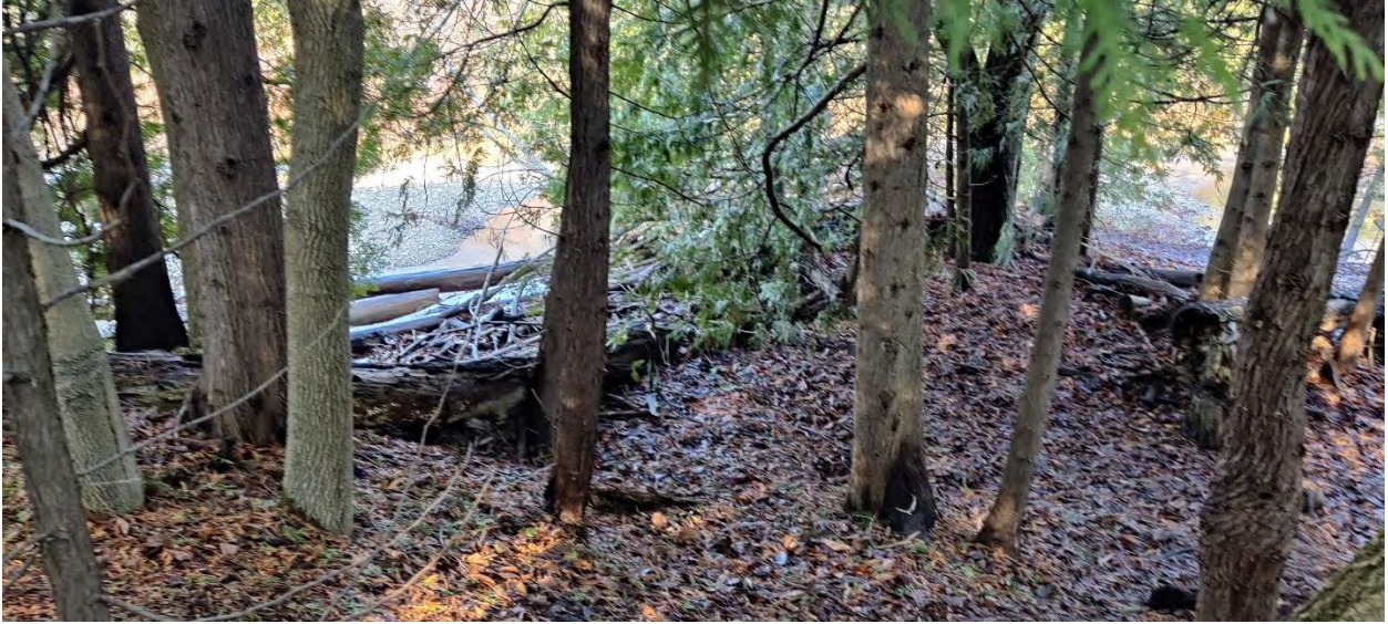
Photo P3: Top of slope conditions in area of Sections X3-X3 to X4-X4 (looking north toward river)
