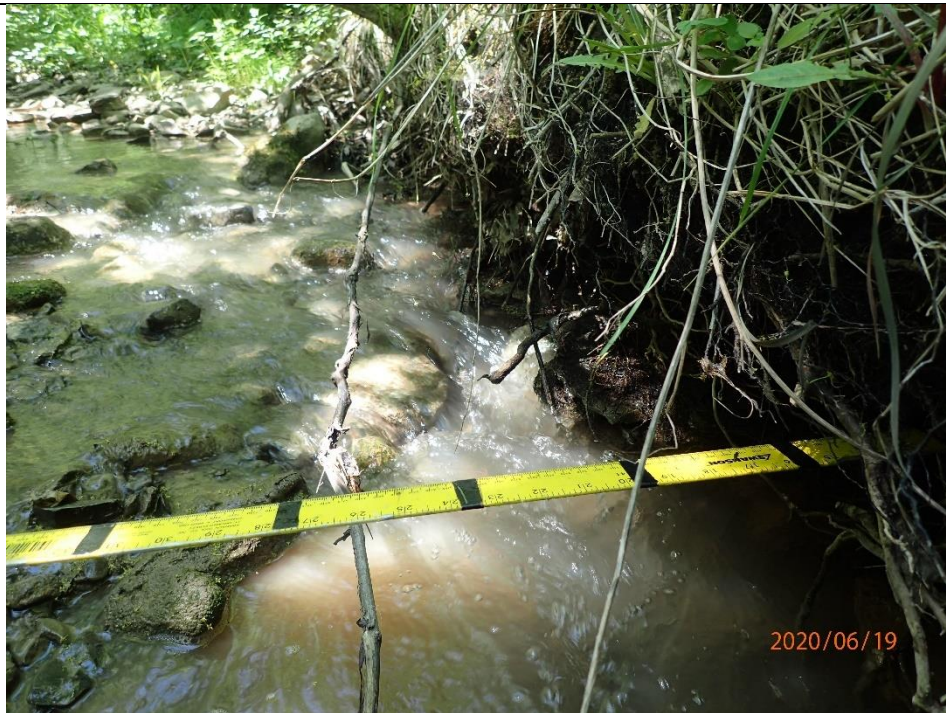
Undercutting was the dominant type of bank failure with undercuts measured up to 0.47 m. Young and old exposed tree roots were common.
