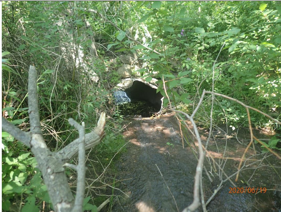
Downstream view at the upstream extent of the reach. Evidence of widening and degradation were the key geomorphic indicators of channel stability through the reach.
