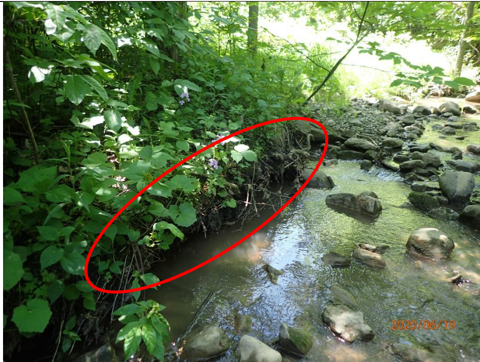
Bank erosion was present through 30 to 60% of the reach and was observed through scouring of the channel banks and undercutting (circled).
