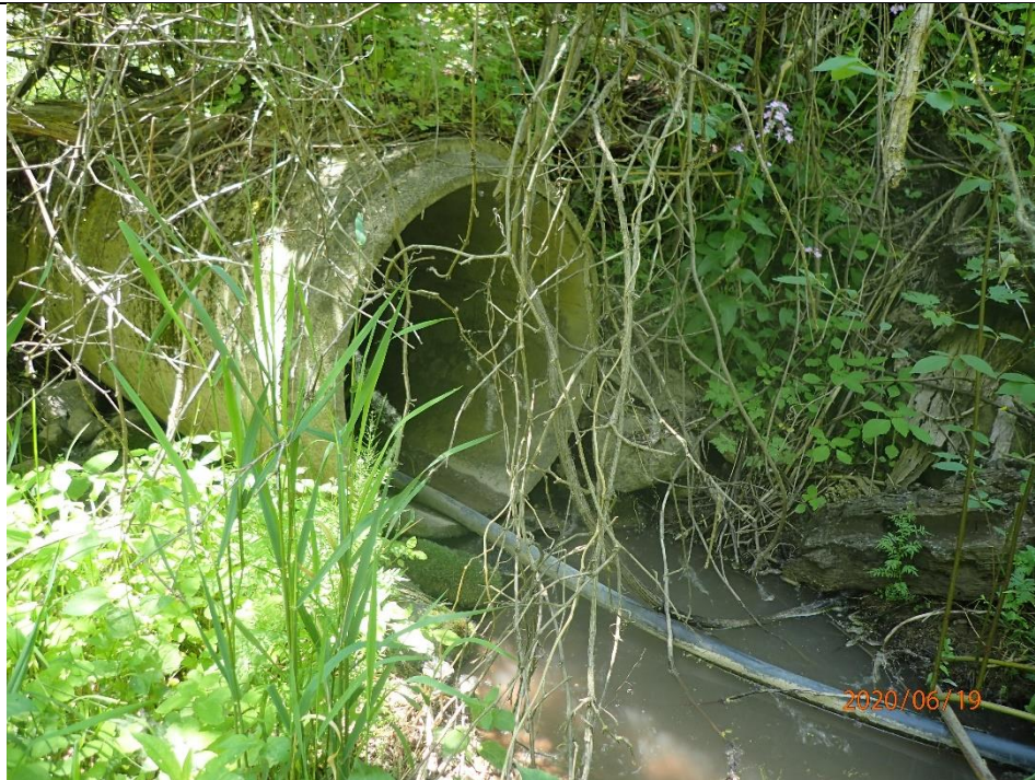
An exposed storm sewer and length of previously buried pipe was located at the upstream extent of the reach. Surrounding bank erosion and undercutting was present. This is indicative of both degradation and widening at this location.
