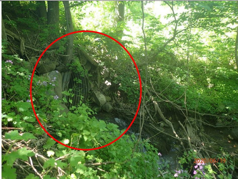
An elevated outfall was observed at the downstream extent of an existing watercourse crossing. A scour pool was present immediately downstream, indicative of degradation.
