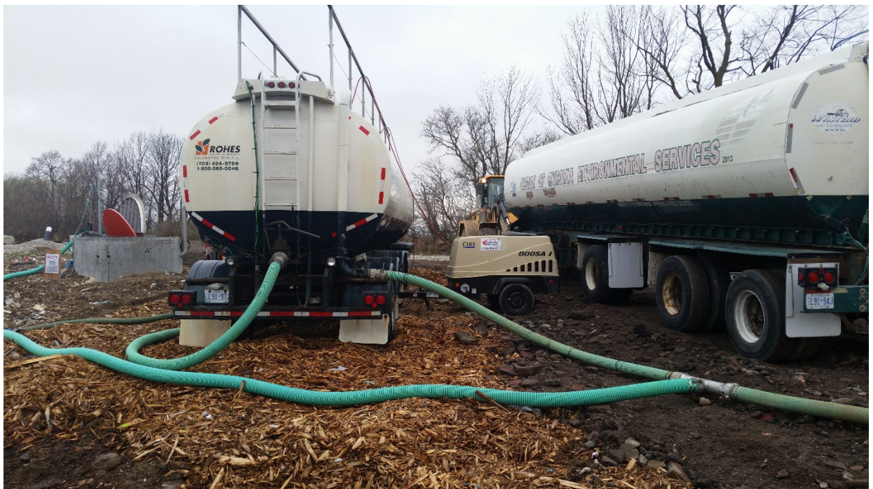
Figure 1. Temporary aeration tankers situation beside landfill cell wet well
